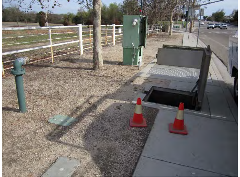
Figure 6-2: Lift Station No. 2 is failing, and should be replaced or abandoned.
