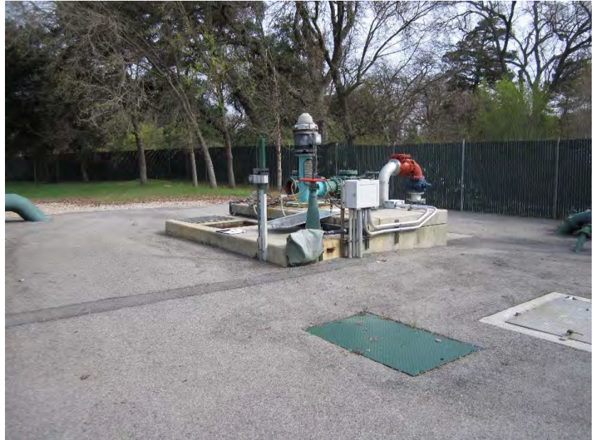
Figure 6-5: A long term plan needs to be developed for Lift Station No. 5, as it is deteriorating
