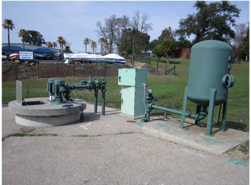
Figure 6-1: Recent modifications to the discharge point of Lift Station No. 1 may allow the surge tank to be removed from this facility.
