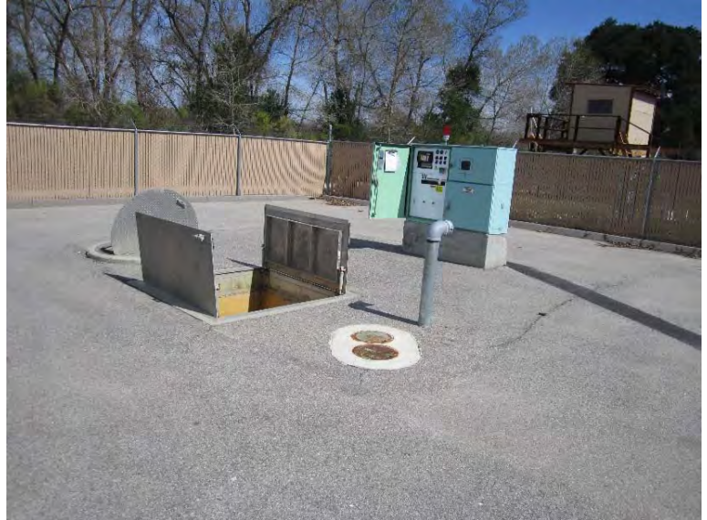
Figure 6-12: Lift Station No. 15 is in good condition.
