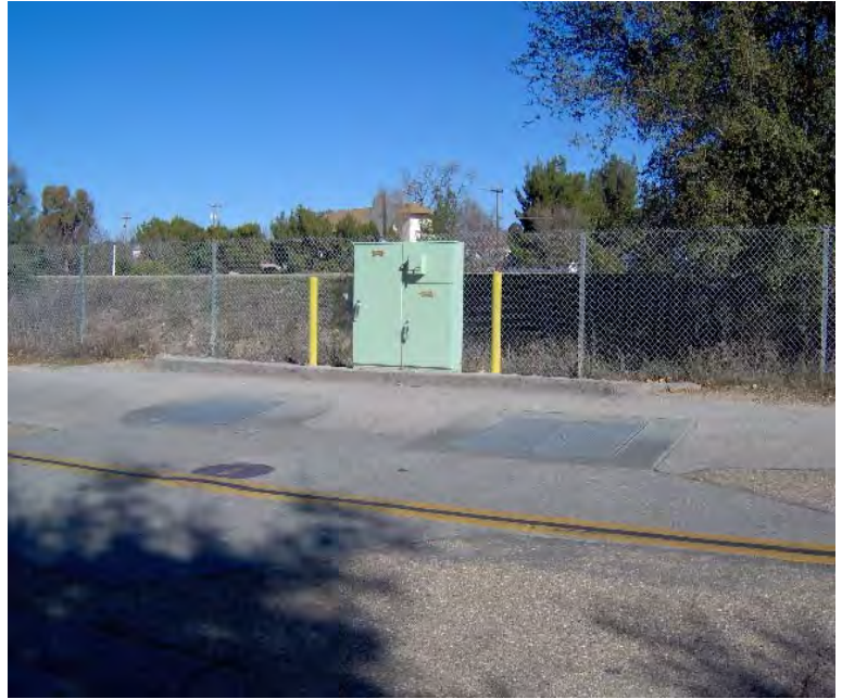
Figure 6-9: Lift Station No. 11 is in a hazardous location, and bypassing the lift station requires shutting down one lane of traffic.
