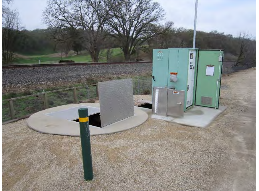
Figure 6-3: Lift Station No. 3 is in good condition, but site improvements would significantly improve working conditions at the site.
