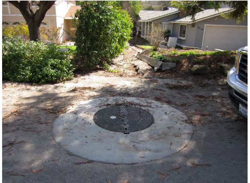
Figure 6-7: The City would like to re-route wastewater from this lift station by gravity to Mananita Avenue, and abandon Lift Station No. 7.
