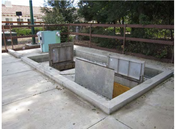
Figure 6-11: The design of the surface features at Lift Station No. 14 creates a challenging work environment.
