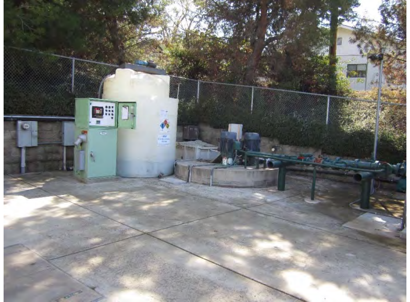
Figure 6-10: The City would like to shorten the alignment of the force main for Lift Station No. 9 to reduce odor complaints and change system hydraulics.
