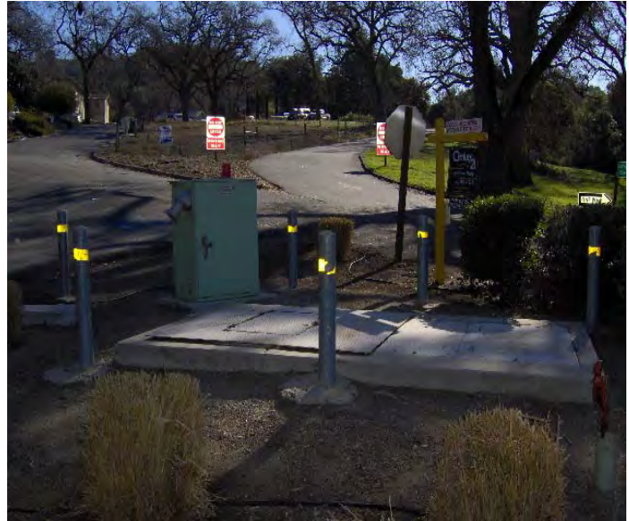
Figure 6-4: Lift Station No. 4 is in good working order. Minor improvements would reinforce the long term reliability and ease of operations at this facility.
