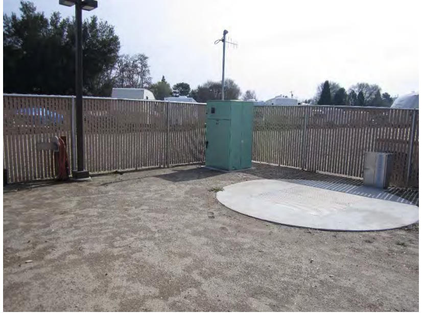
Figure 6-6: Lift Station No. 6 was recently rehabilitated, but due to budget constraints, some site improvements were omitted from the project.
